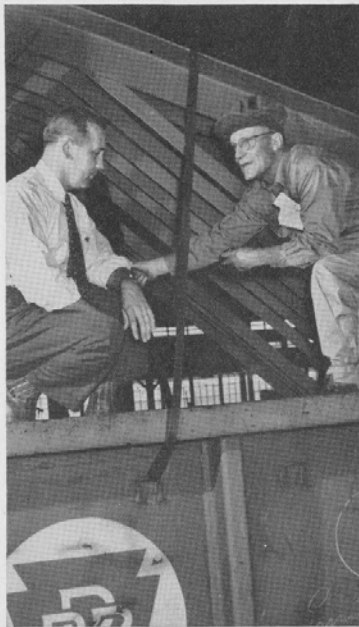
E. R. Buchwalter of Dresser-Stacey, who calls him PRR's "best salesman," joins Mr. Cleveland in inspection of roof trusses
